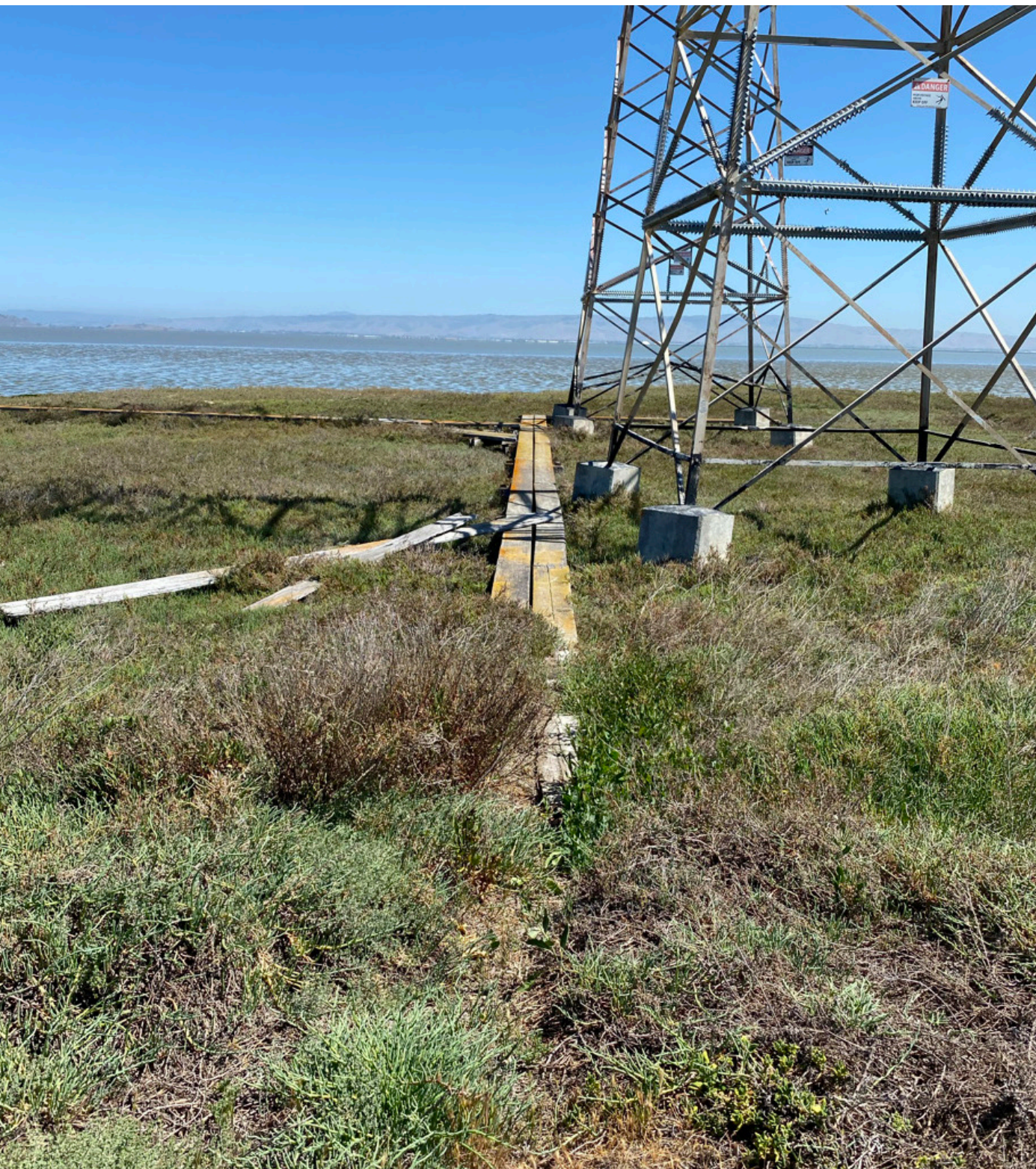
Figure 2. Existing boardwalk requiring replacement.
