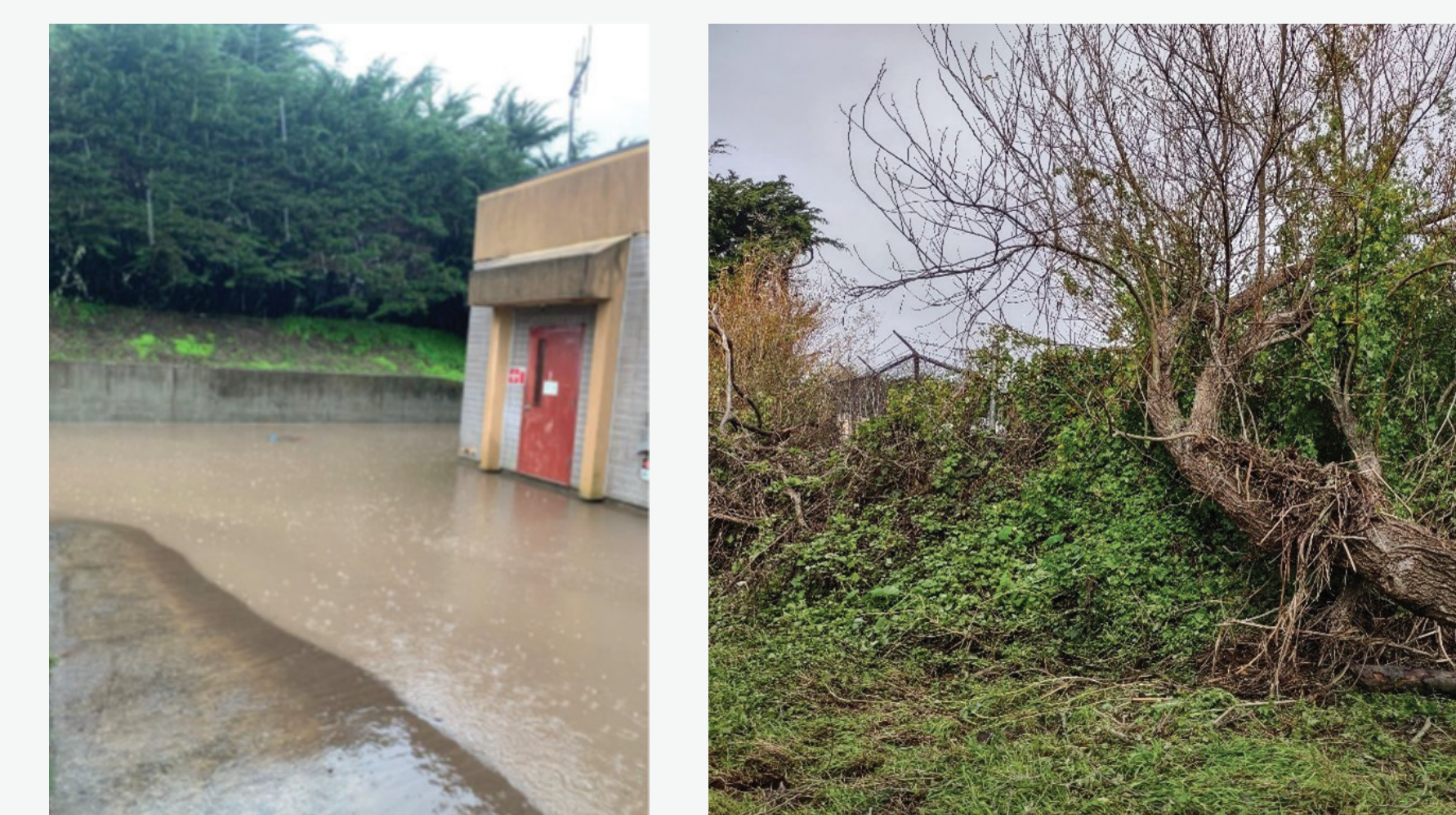
Figure 6. Flooding at Mechanical Building No. 1 (left); Low-lying location south of berm overtopping (right)
